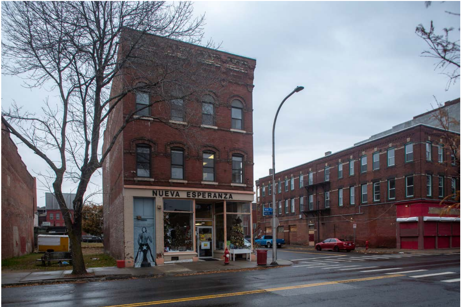
View from the southeast showing exposed party wall. Photo by Zachary Violette
